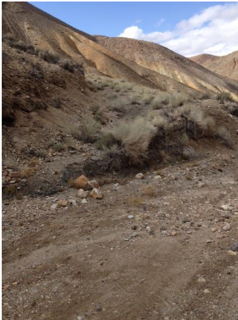
Photo 3. Junction of Road #4 with Wildhorse Canyon road in the wash bottom at waypoint 90 looking NW. Last few feet of Road #4 are washed out. Although brush is growing on Road #4, it is clearly a bladed (mechanically constructed) road. Road #4 leads to a mining prospect with constructed drill sites.
